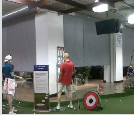
Retail - fire curtain in mid position
